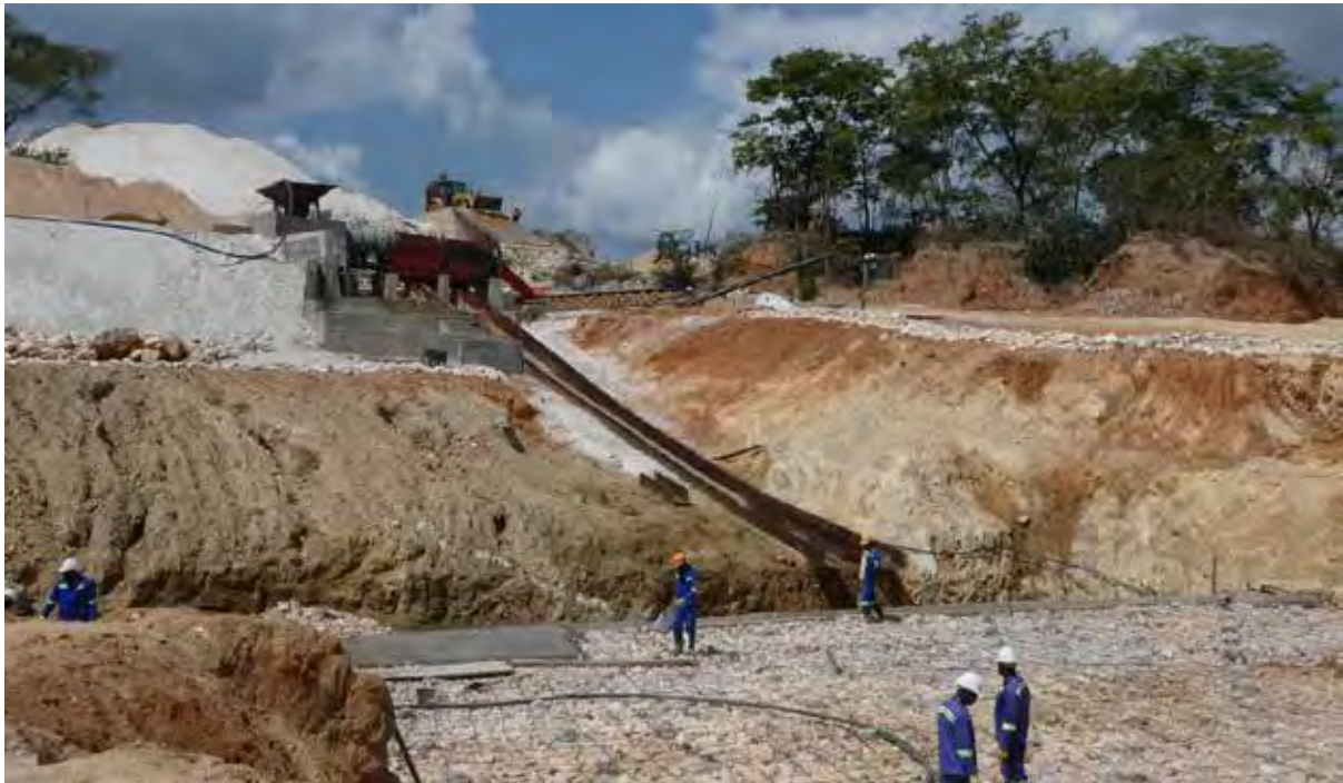
Figure 7: Construction of the processing plant at the Naipa mine owned by French and Mozambican partners.
