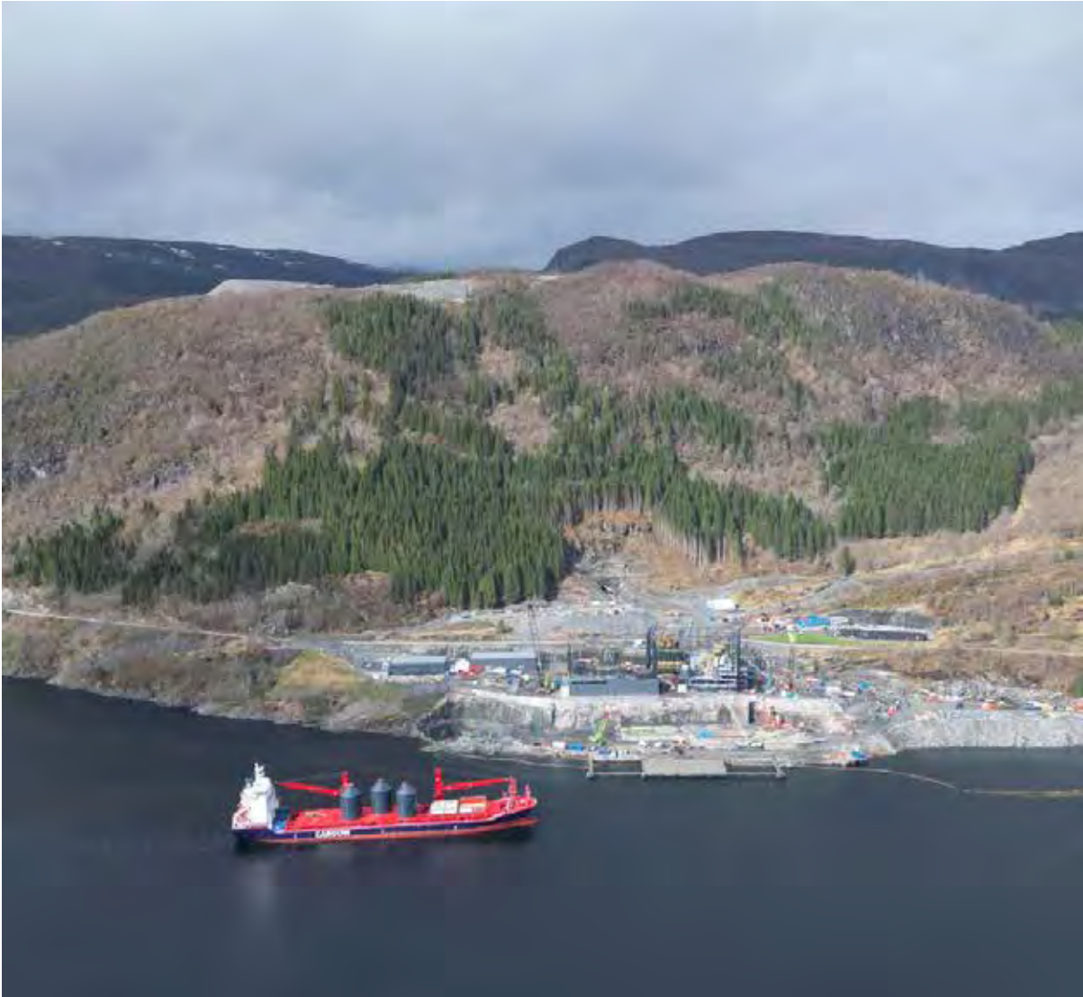
Figure 3: Ongoing construction at the Engebø rutile and garnet deposit. Production ramp-up is planned for Q4 2024, eventually reaching 35 kt TiO 2 per year. Photo: Nordic Mining.
